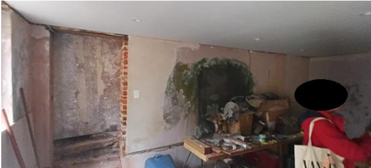
Figure 7: Ground floor storage space at the far end of the south-eastern wing
